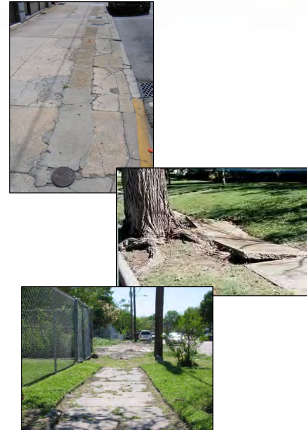
Examples of poor pavement quality
